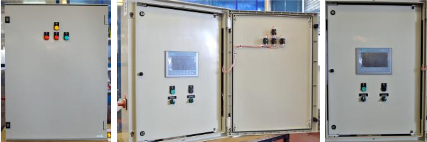
The Sub-Master Control Panel
